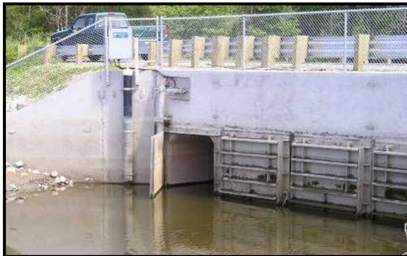
Figure 4-2. McElroy Slough Automatic Regulating Tidegate, “Aberdeen” style gate, open at a -2.7 foot tide event (County owned tidegate complex).
