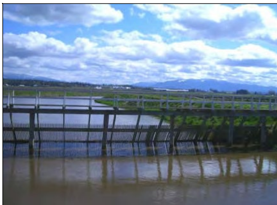
Exhibit 2-3. Trash Rack on Big Indian Slough
