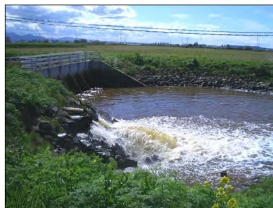
Exhibit 2-4. Tide Gates and Activated Pump
